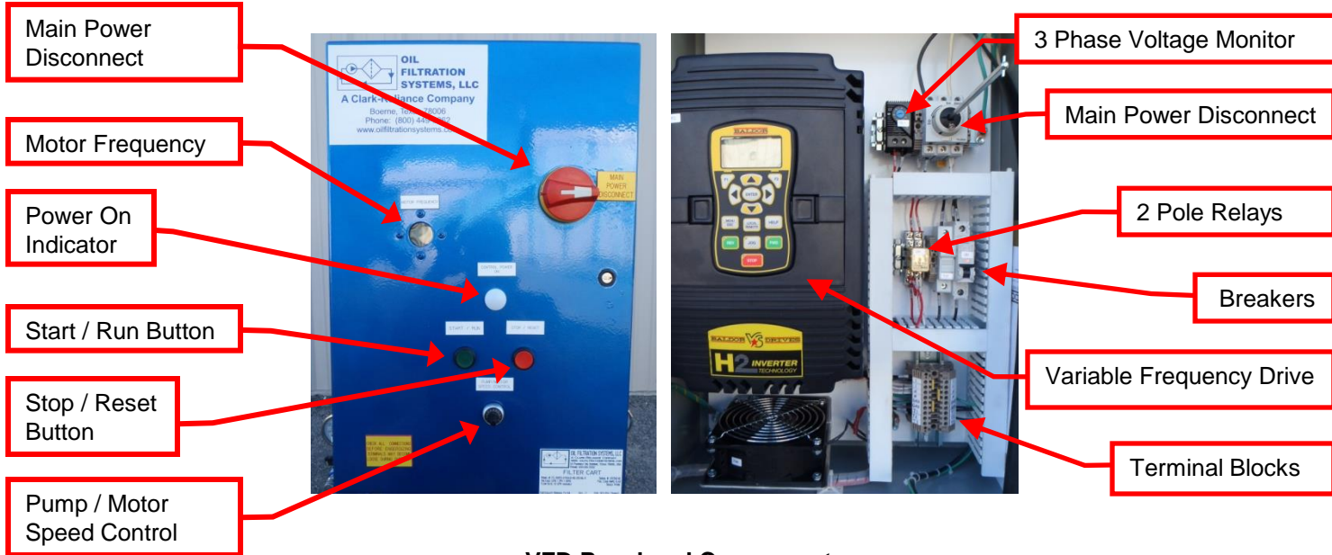
VFD Panel and Components
